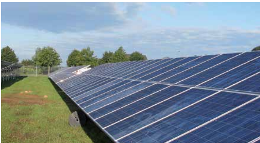
Domsühl - Germany System: 1 MW | N-Rack System - Screw foundation
